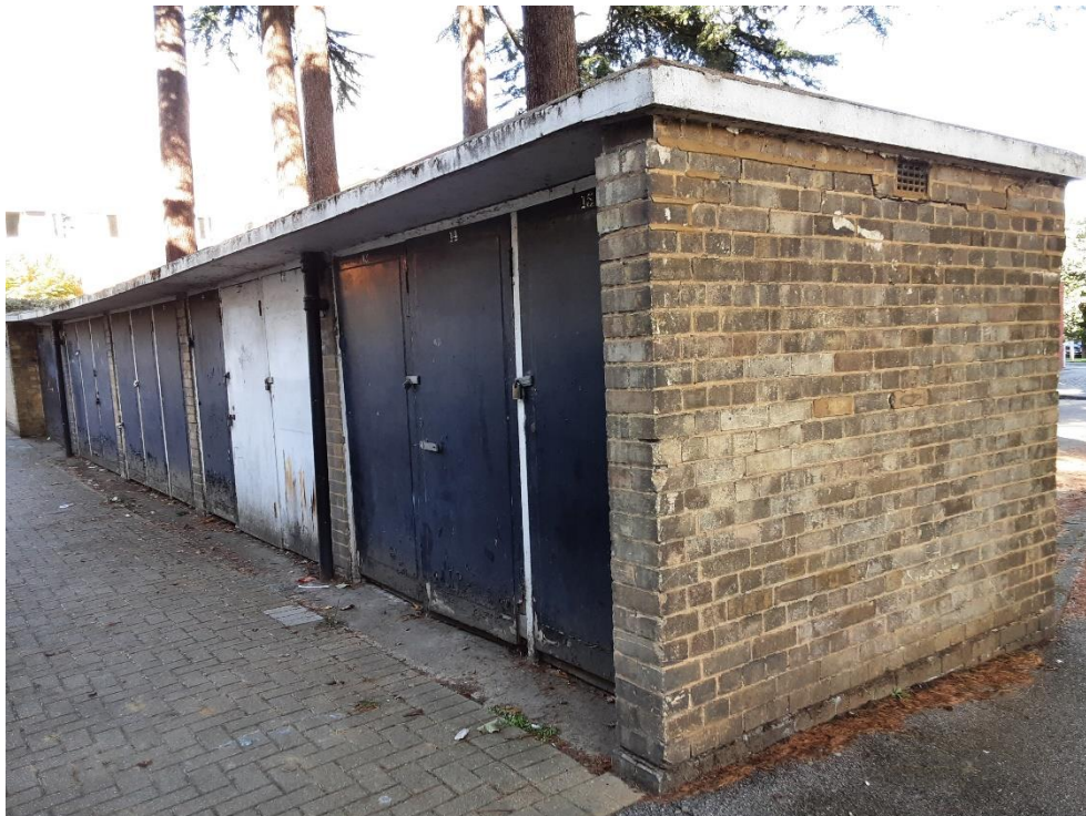
Photograph 4: Storage units, building B2
