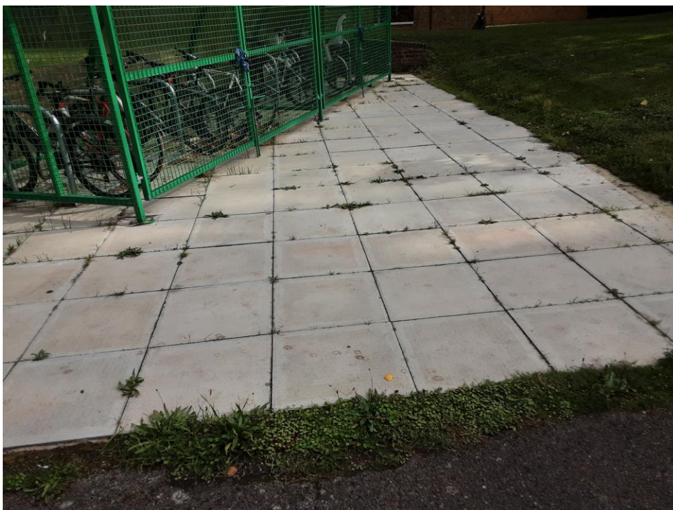
Photograph 2: Vegetation growth between paving slabs within Site 4
